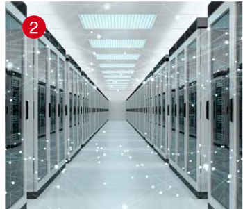
2 Hot / Cold aisle containment
