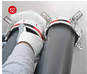
12 Piping and ventilation
