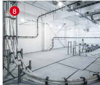
8 High-voltage cabling supports
