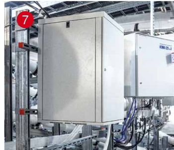
7 Equipment supports and platforms
